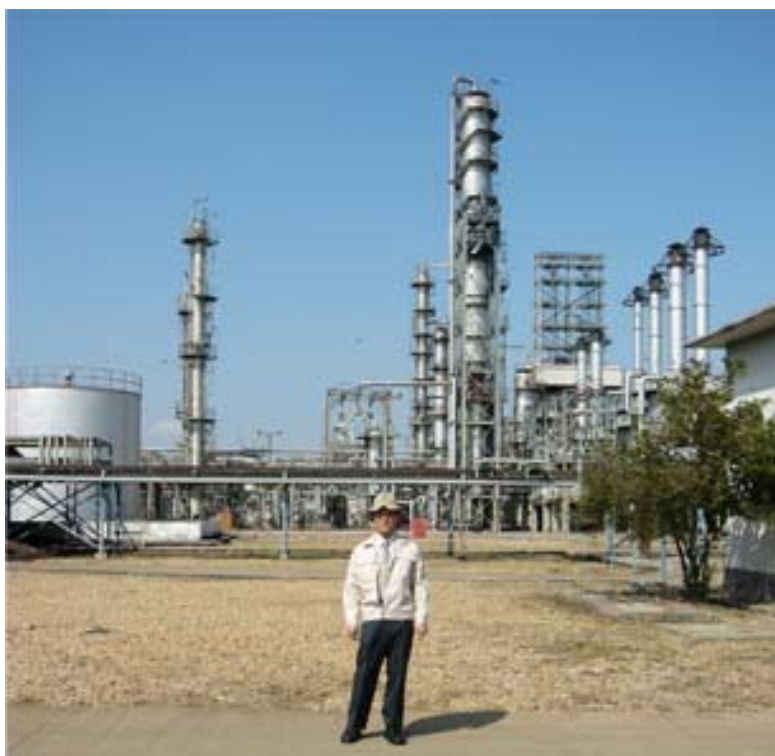
Photo -3-1 Refinery Tower of Thanbayakan Oil Refinery (Atmospheric Distillation Plant, etc.)
