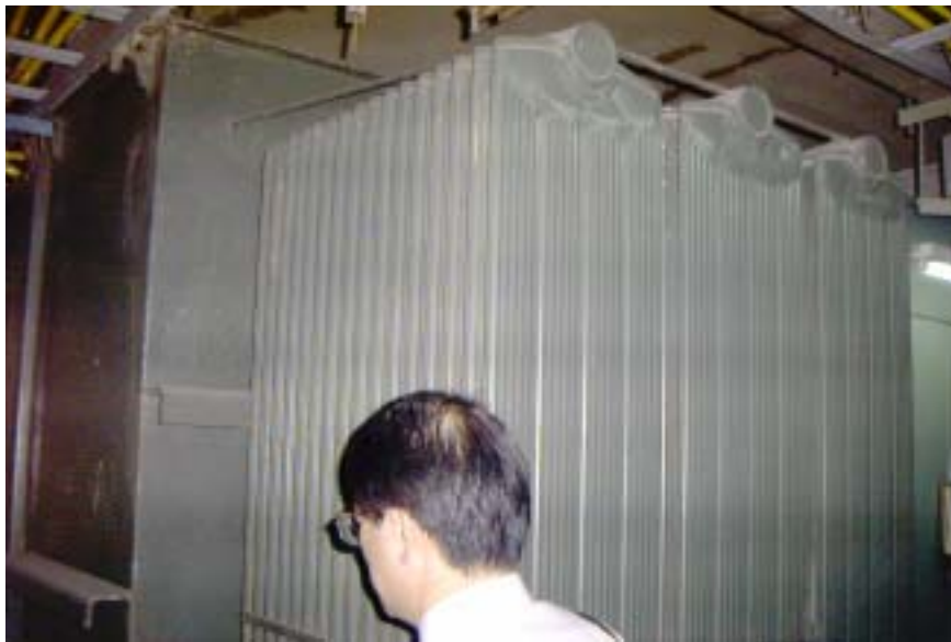
Figure V-4-16 Old Excessive Transformer
