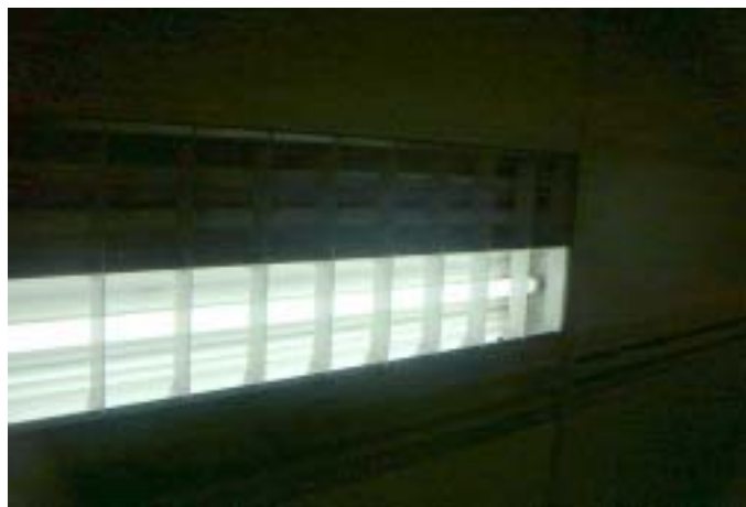
Figure V-4-5 Two-Lamp Fluorescent Lighting with One Lamp Off
