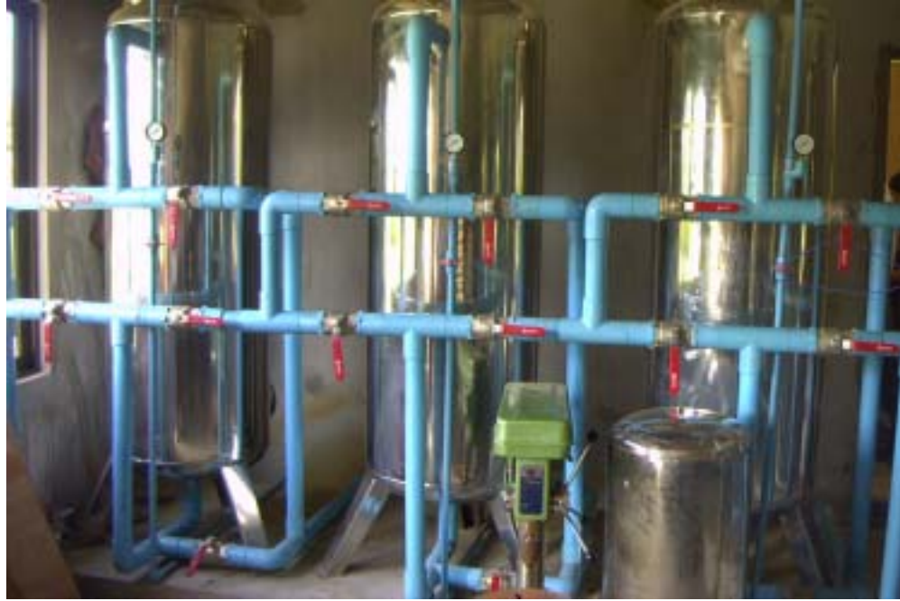
Figure III-4-4 Water Processing Facility
