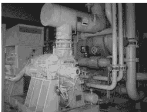
Photo 1 PG Brine Chiller
