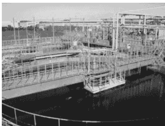
Photo 2 Full View of the Effluent Treatment Plant
