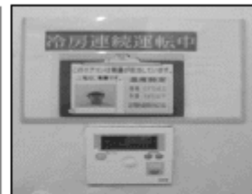
(4) Management values and responsible people are indicated above the air conditioning switch.
