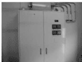
Fig. 9 Control Board of Exhaust Fan
