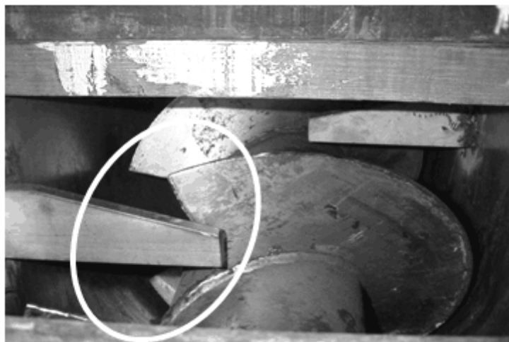
Photo-1 Measure on the conveyer
