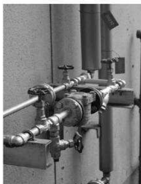
Photograph 8 Steam Trap and Number Tag Setting Condition
