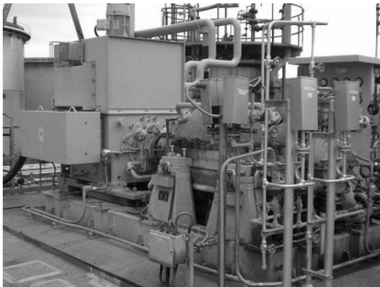
Fig. 5 Equipment Exterior View (New Inverter Motor and Existing Butane Gas Compressor)
