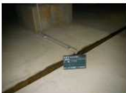
Photo-9 Before drain piping repair
