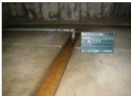
Photo-7 Before drain piping repair
