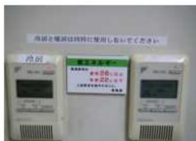
Photo 5 Air-con switch sticker
