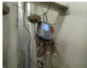
Photo-3. Thermocouple data logger
