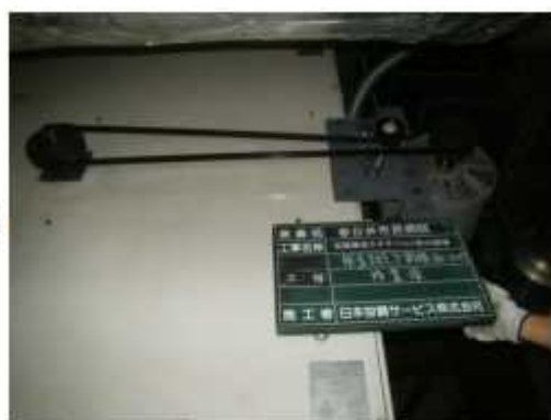
Photo-18 Air-conditioner fitted with flat belt
