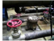
Steam Trap for (Fuel Oil) Heater (TLV-made, 2-1/2" Free Float Type)
