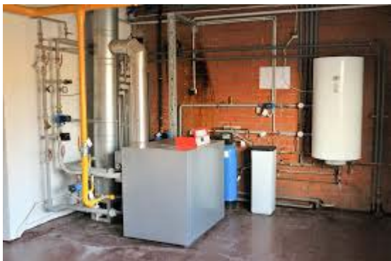
Natural gas/oil water boiler
