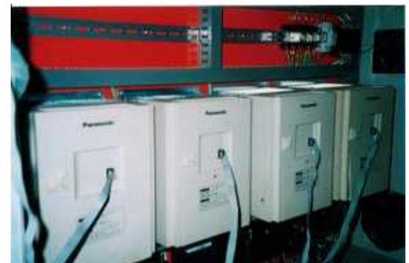
Variable speed Drive (VSD) control chilled pump and cooling tower pump
