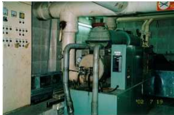
The water chiller system
